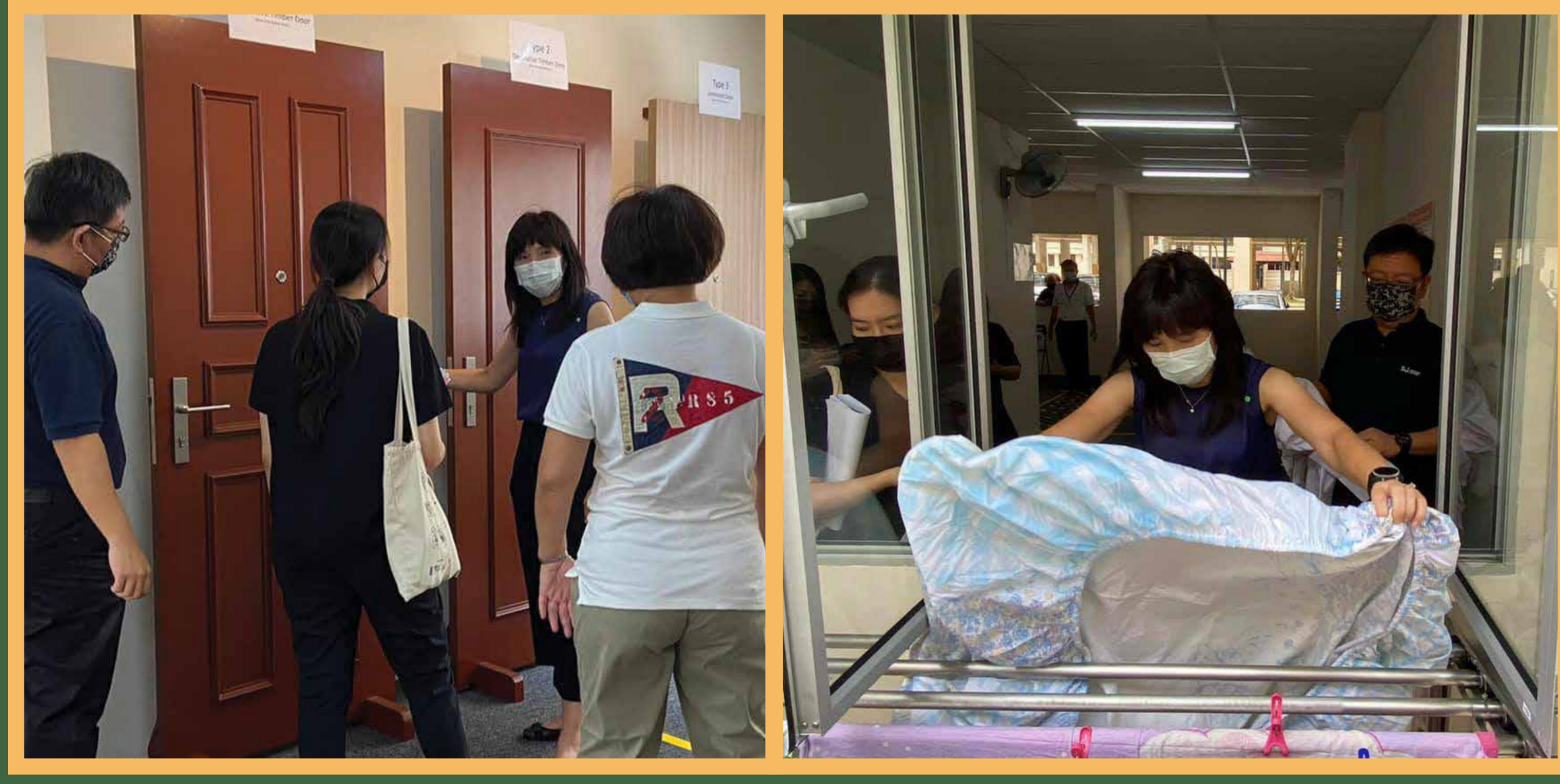
Home Improvement Programme was safely carried out in 6 phases across 72 blocks during the pandemic. Many partners worked tirelessly to deliver quality improvements in a timely manner
