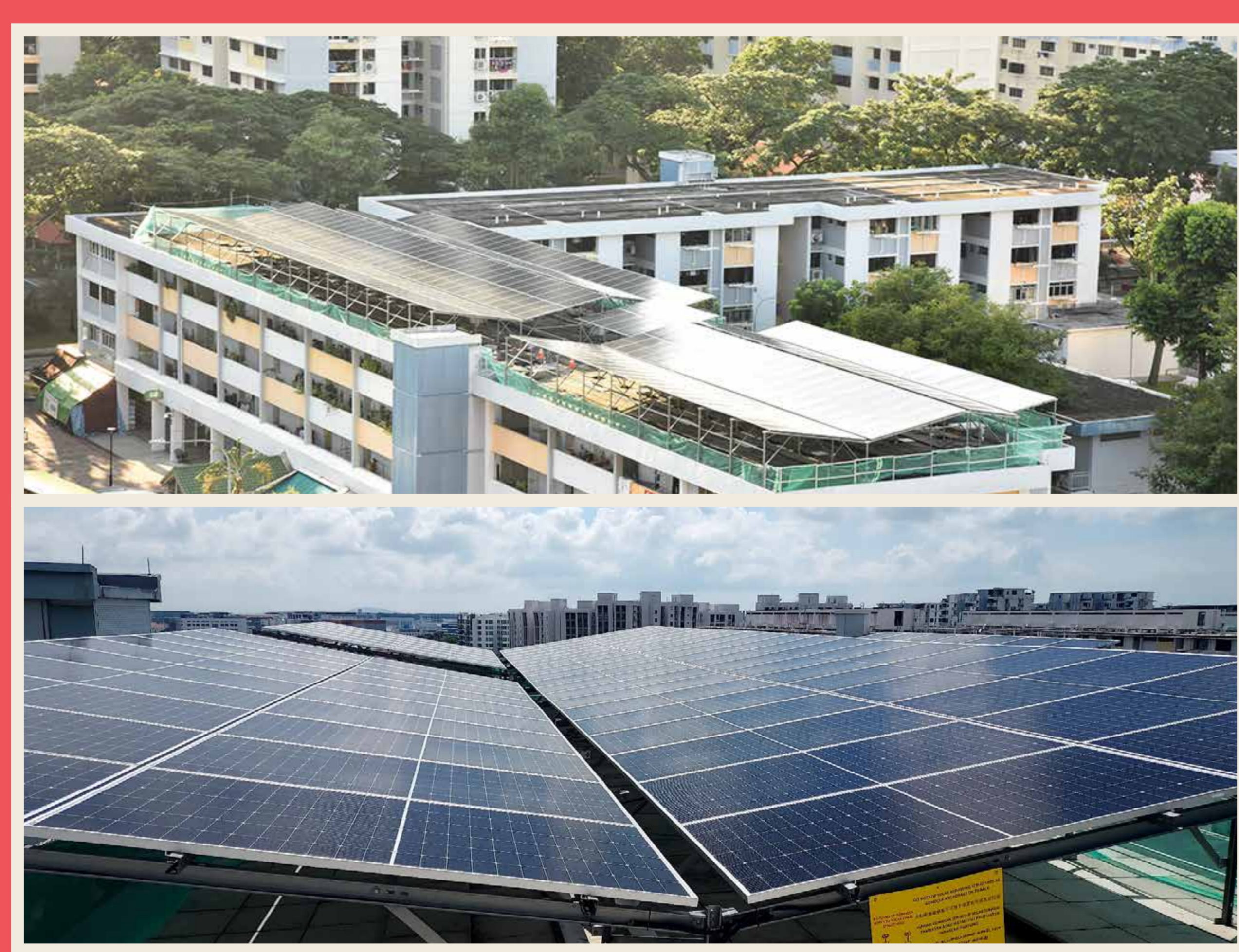
On-going installation of solar panels across East Coast for a sustainable town
